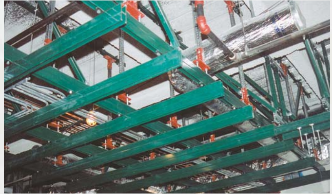
Multi-rail support system with Telespar drops.
